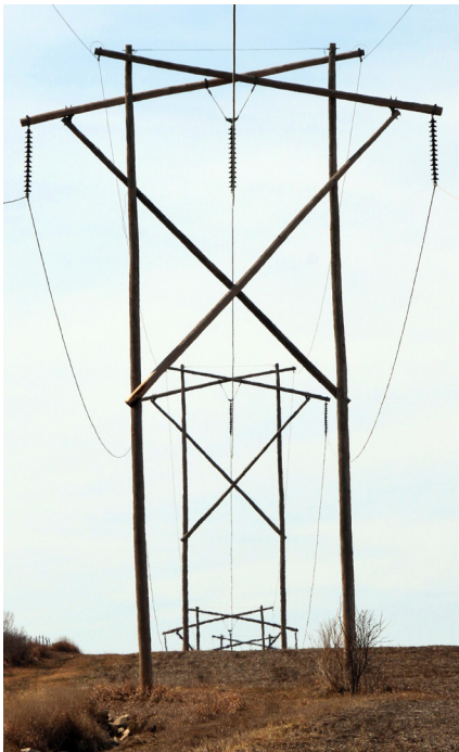
Aging spar-arm structure, shorter service life due to eccentricities of loads and sub-standard framing.
