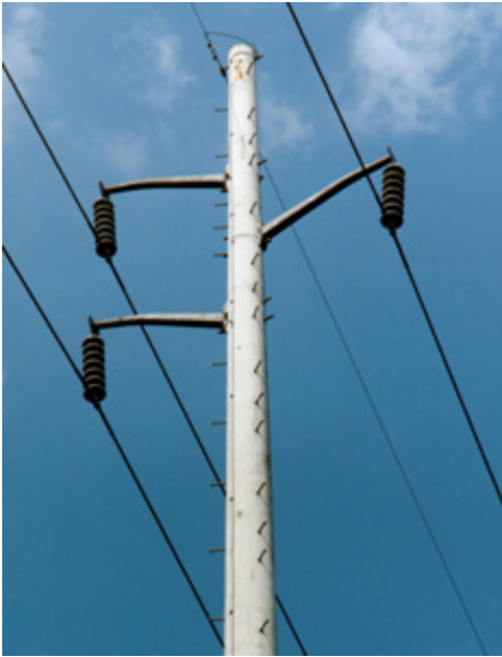
Galvanized steel davits on spun concrete pole
