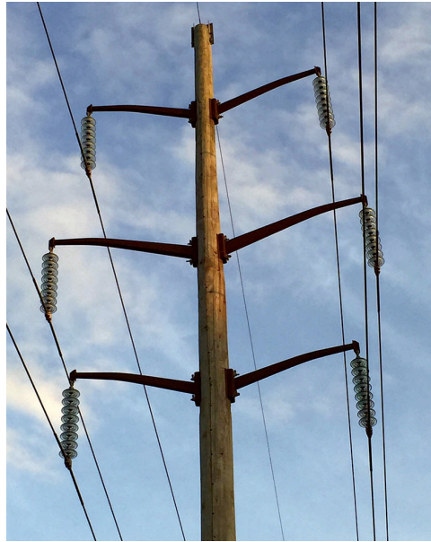
Weathering steel davits on round wood pole
